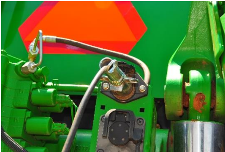
Electrical connector inserted into tractor.
